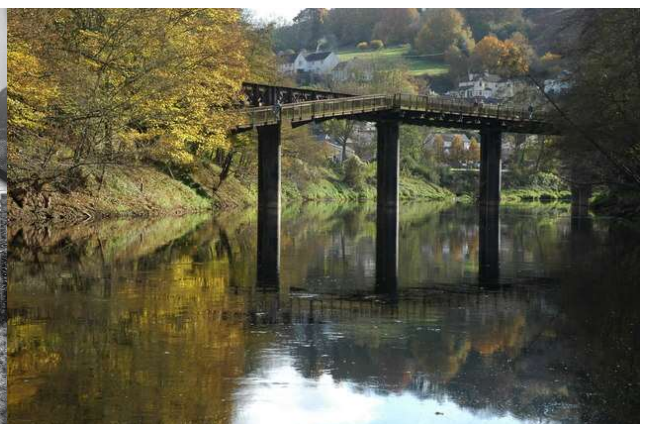
Penallt viaduct between Redbrook-on-wye station and Penallt Halt ( Phillip Halling CC BY-SA 2.0 )
