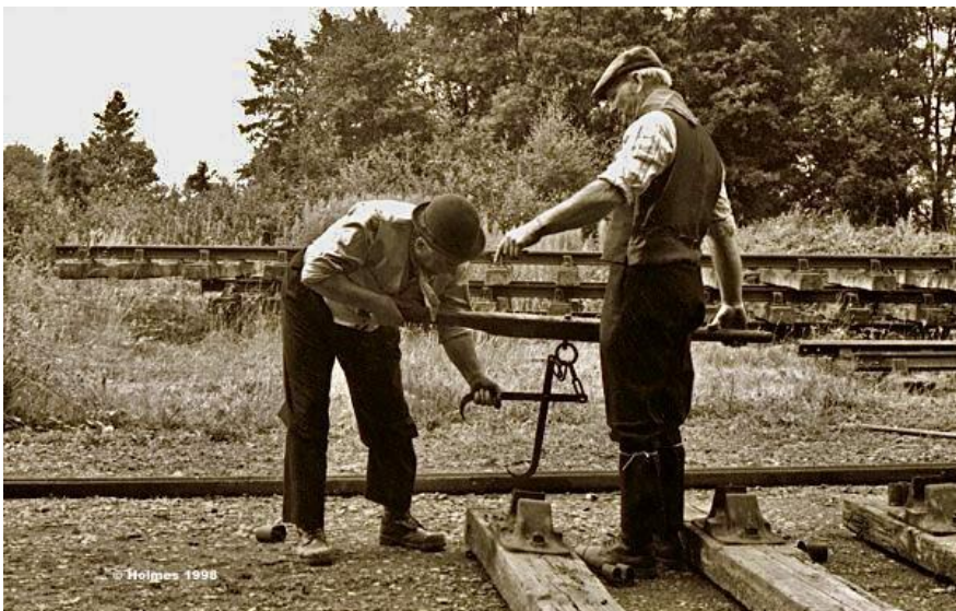
Fitting one of the two sleeper nips for final positioning of the sleeper.
