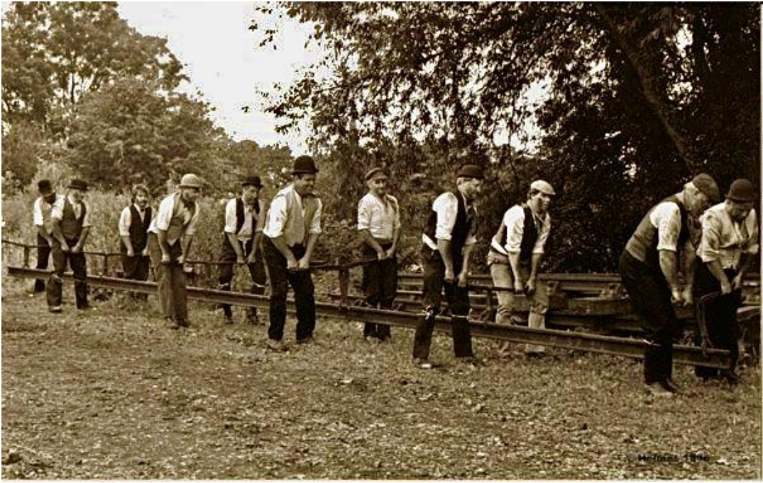
12 men manoeuvring a length of rail. The rail weighs approximately 30 kg per metre. It is important that the navvies walk in step to avoid dropping the rail.
