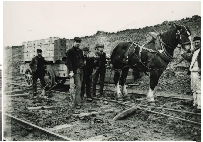
Navvies and boys at work in a shallow cutting at Grendon-Haddenham, Buckinghamshire, circa 1903. The rails are not the permanent way, but temporary tracks laid by the contractor. Both horses and locomotives were used to pull the large number of tipping wagons required to move the enormous quantities of earth between cuttings and embankments. (Record Office for Leicestershire, Leicester and Rutland)
