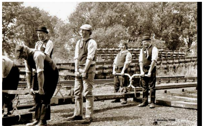
Using sleeper nips to manoeuvre a sleeper into position with the chairs fitted.
