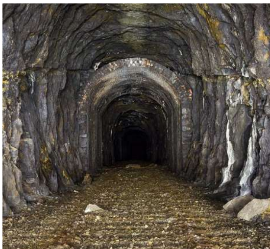
Tidenham tunnel. Unlined section followed by brick-lined section ( Graeme Bickerdike – Forgotten relics )
